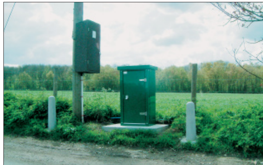
Far left: Poorly sited telecommunications mast
