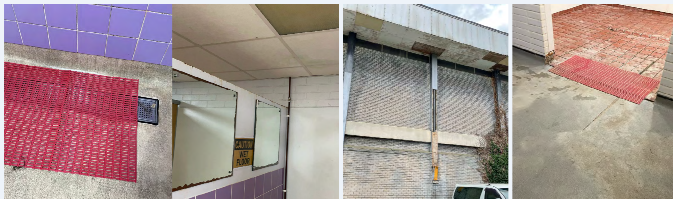
WET CHANGING ROOM FLOOR CONDITION | LIGHTS OUT | MIRROR DAMAGE | EXTERNAL CONDITION WATER DAMAGE | DAMAGE | DRY CHANGE TILE & FLOOR DAMAGE
